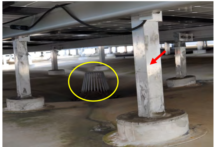
Figure 10 PV panels extended over this roof drain (yellow oval), thereby making it difficult to check for dogging and removal of debris. The red arrow indicates a rail support post.
