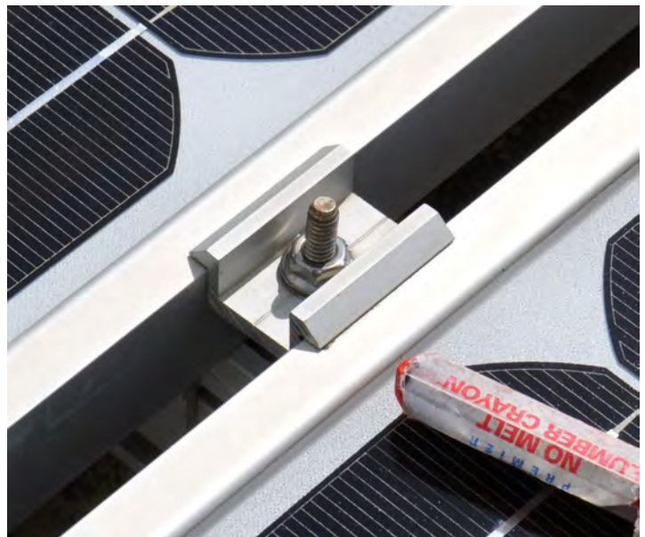
Figure 13. View of a PV panel clip after the 2017 hurricanes. Although there was no apparent loosening of the nut, the bolt could be wobbled with finger pressure. A loose nut such as this is susceptible to further loosening and loss of the clamp's ability to keep the panels in place.
