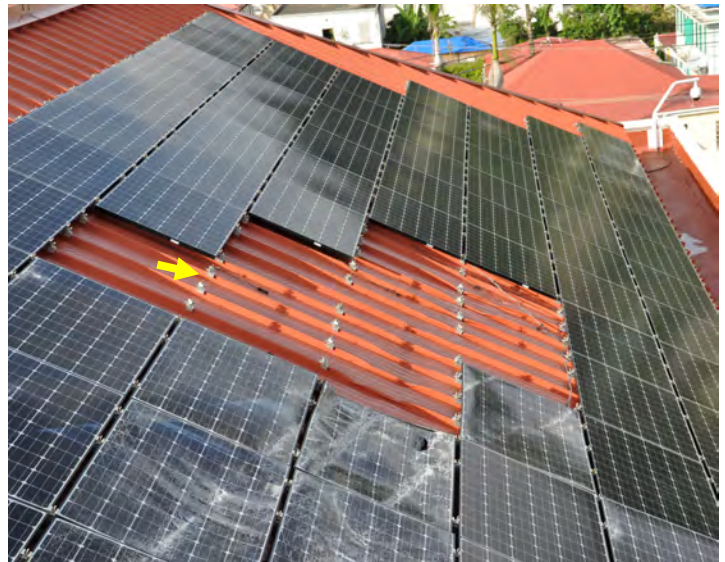
Figure 12. These PV panels were attached directly to the standing seam ribs with panel clamps that were attached to external seam clamps (yellow arrow). Note that several panels in the foreground were damaged by wind-borne debris (reportedly a collapsed antenna).
